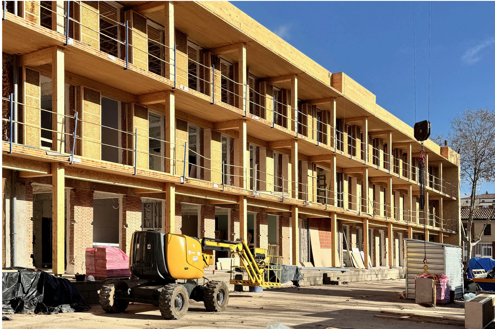
Top: Overall view of the main building elevation, with EcoCocon wrapping and additional balconies constructed from CLT and glulam frame
